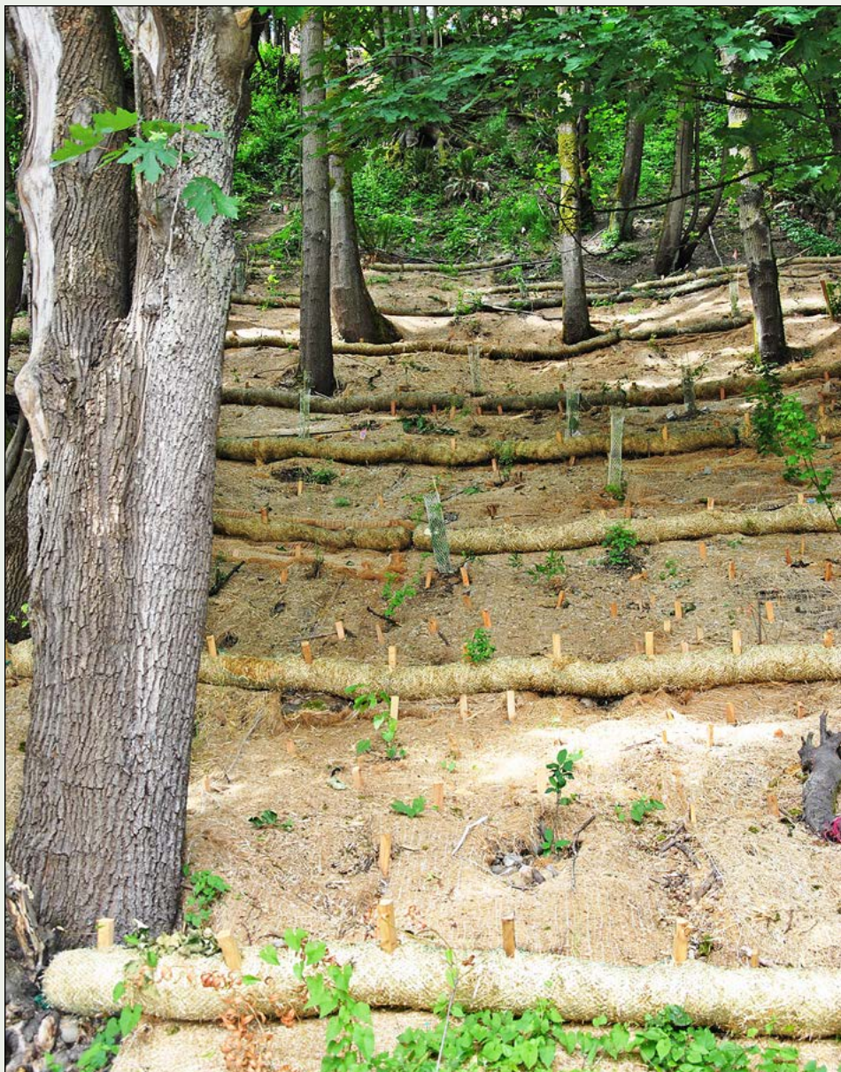
Erosion control and plantings along the Schuster hillside in between existing trees. Photo Courtesy City of Tacoma
