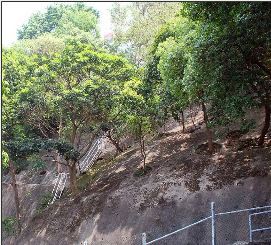
Many engineered slopes in Hong Kong have trees planted on them inside small planters.
