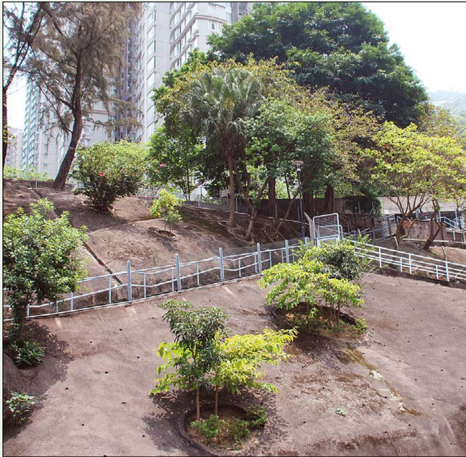
A substantial amount of “shotcrete” has been laid to aid in slope stabilization in Hong Kong. Photo by Jeff Shimonski
