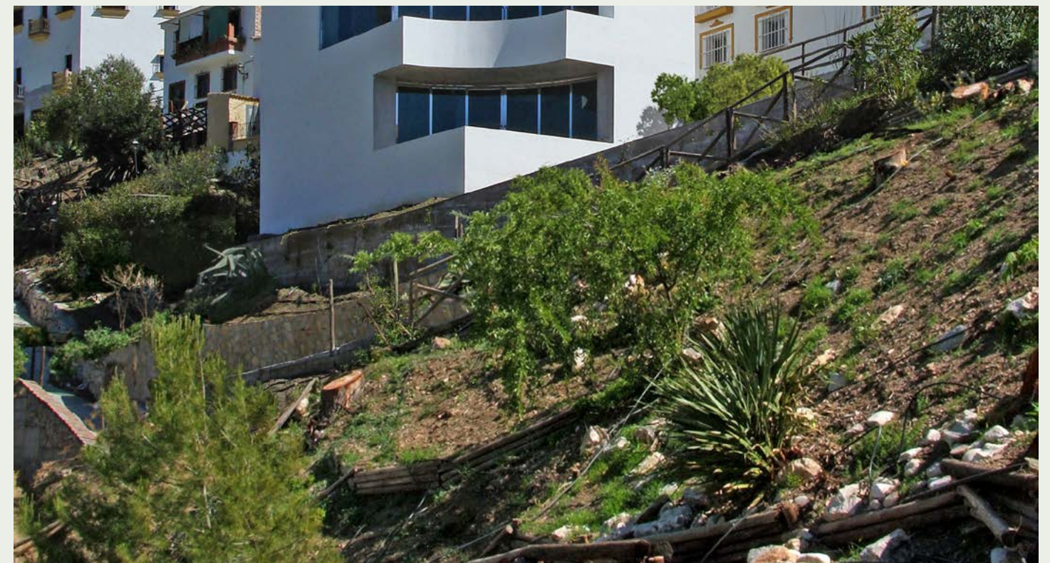
The existing slope condition in Totalán park in Malaga, Spain. Photo by Sven Roettger
