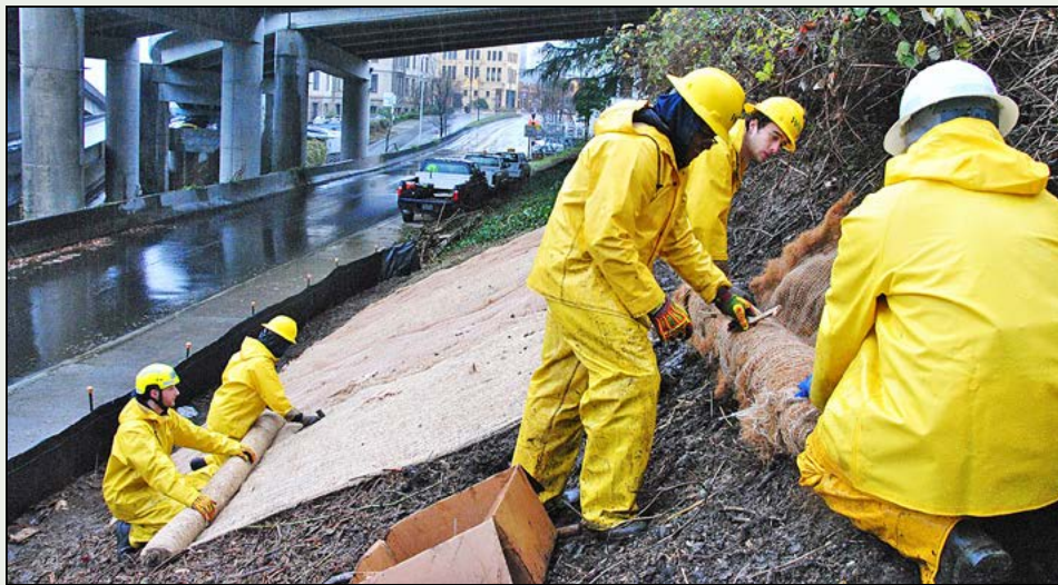
Washington Conservation Corp crews hard at work installing erosion control blankets on Schuster Slope. Photo Courtesy City of Tacoma
