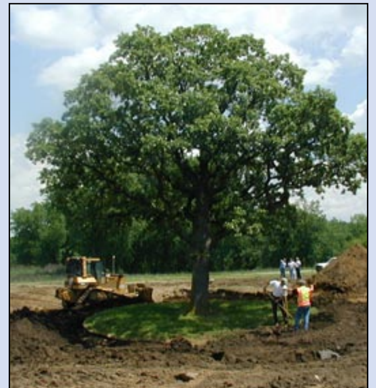
This new site was carefully engineered so the tree would set with the same north-south direction, the same tilt, and the same ground slope in the immediate area. Also, topsoil was trucked over from the original spot.
