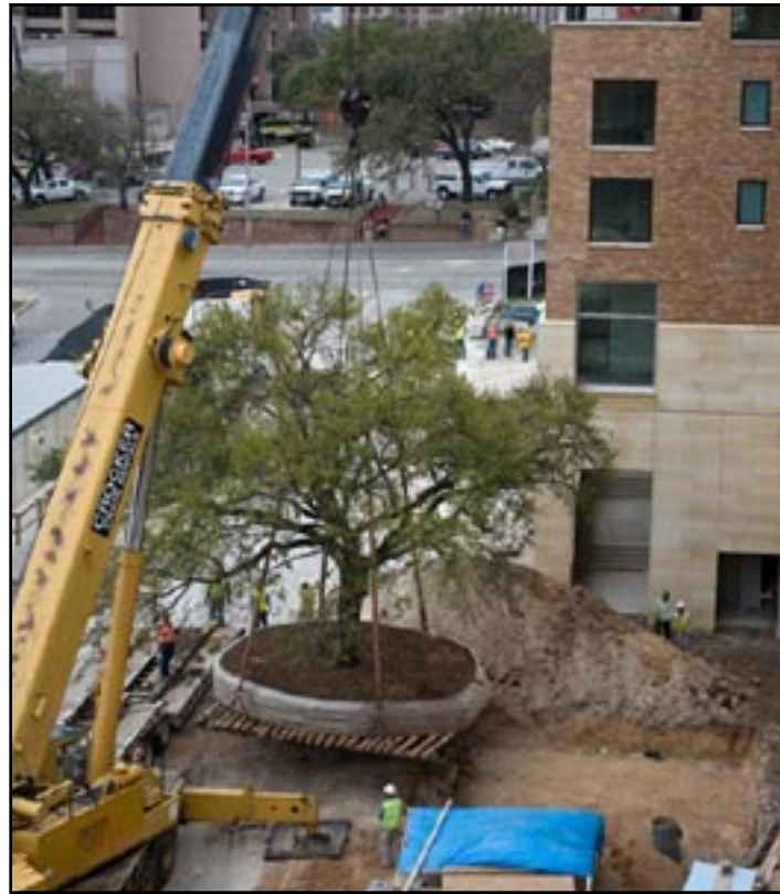
A 24-inch DBH (61 cm) southern live oak gets transplanted to the grounds of the Executive Education and Conference Center at the University of Texas at Austin in April 2008. Photo by Jim Lincoln
