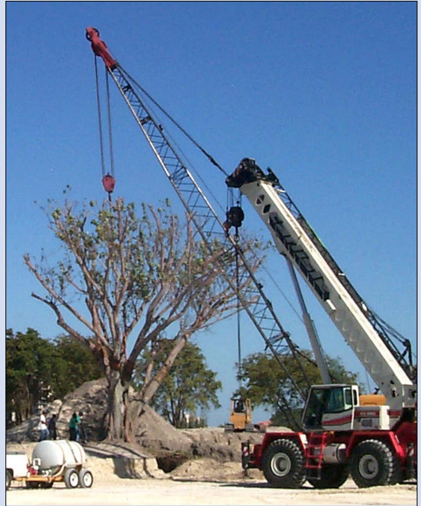
An 80-ton crane was needed to move this bo tree ( Ficus religiosa ) in Jungle Island in Miami, Florida. The canopy had to be “topped” because the staff was unable to pass the three cables from the spreader bar through the dense foliage. The compression damage from the tree straps initiated aerial roots which were then guided down telephone poles to aid in supporting the tree in high winds. Photo by Jeff Shimonski
